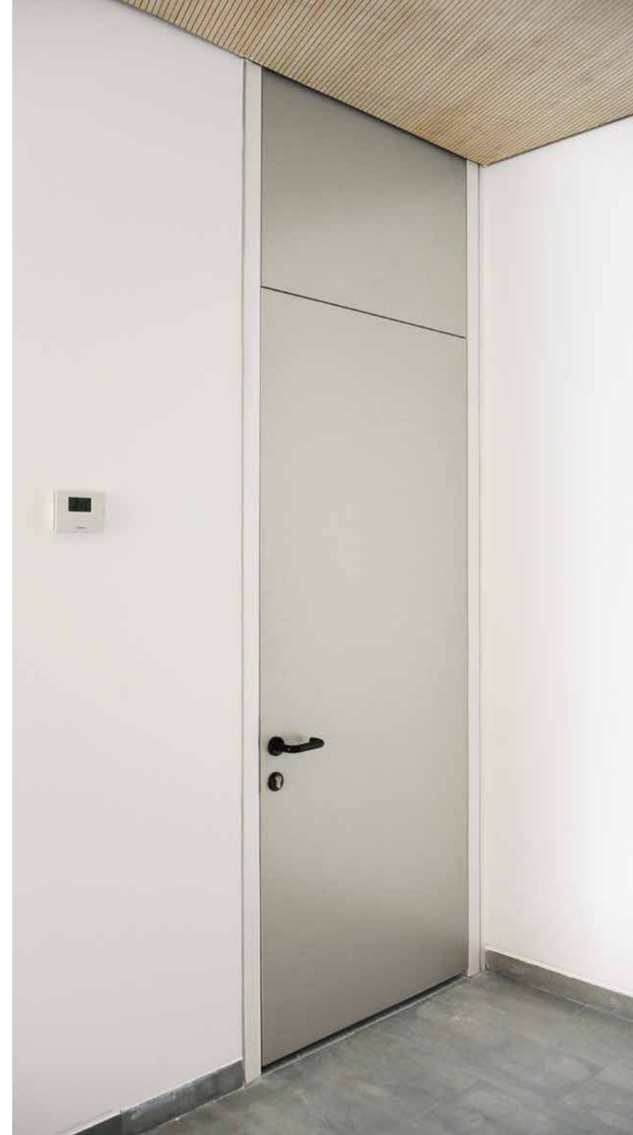
Dettaglio porta con sopraluce cieco a filo Detail of the door with with a blind overpanel transom
